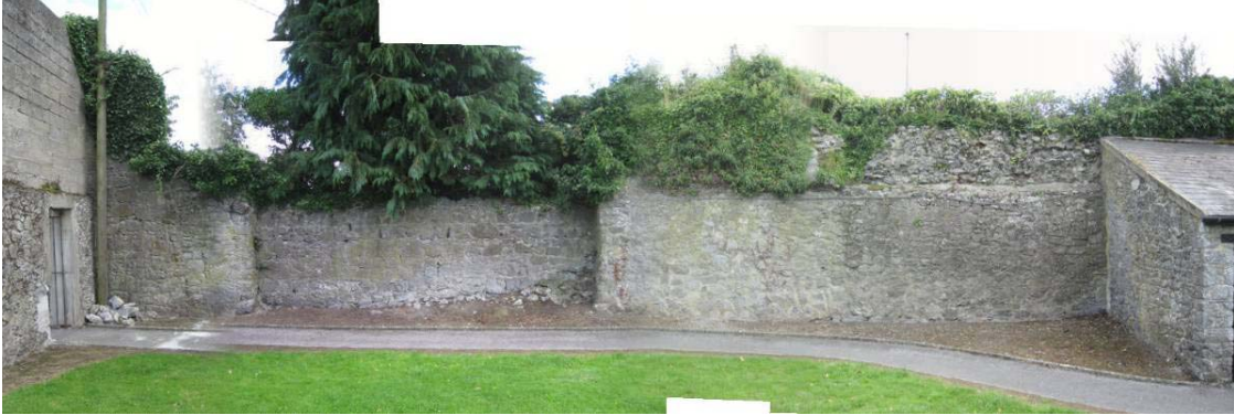
Fig. 14 Section B-2010, (Gazetteer 2.37) North side. Before conservation.
