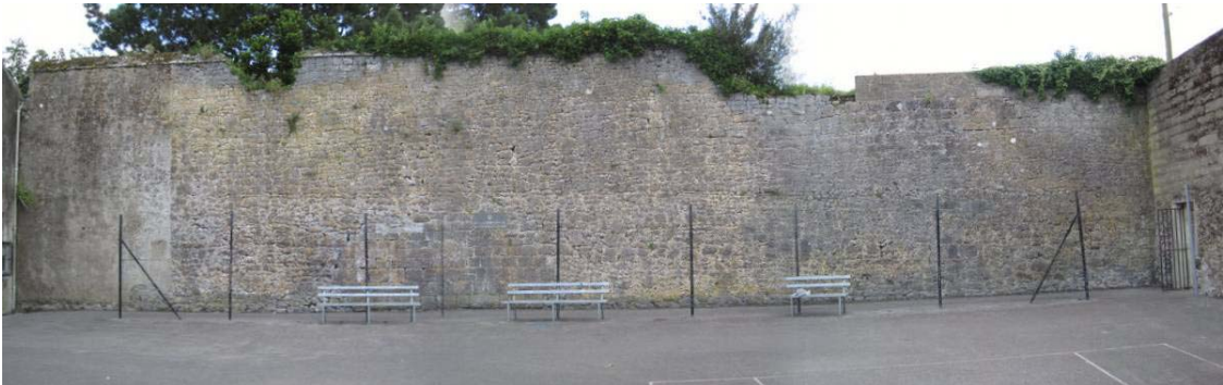
Fig 19 Section B-2010, (Gazetteer 2.36) North side. Before conservation.
