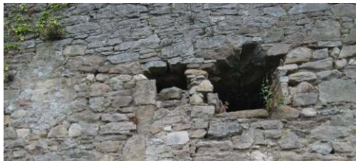
Fig 1 Prior to conservation
