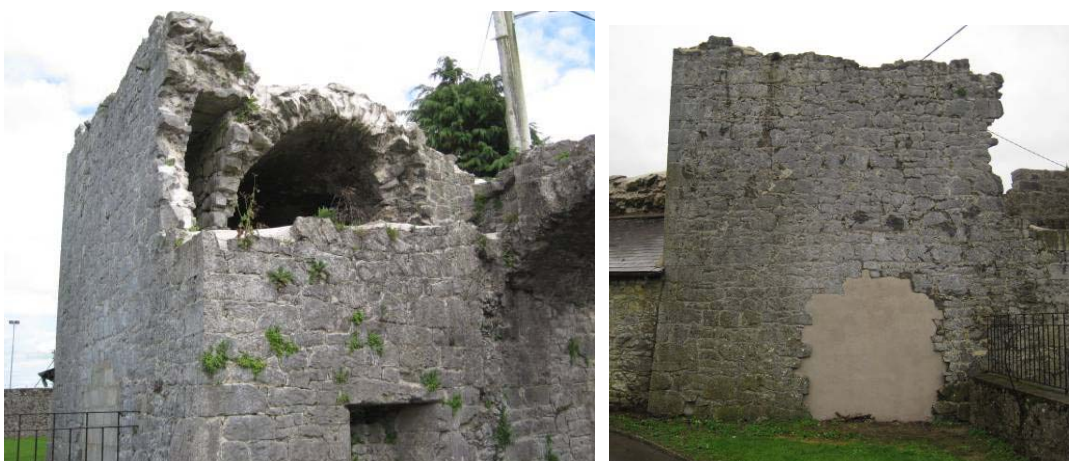
Fig. 9/10 Section A-2010 (Gazetteer 2.01) Vegetation on Currikeen Castle, and after conservation, see also rendered block area.
