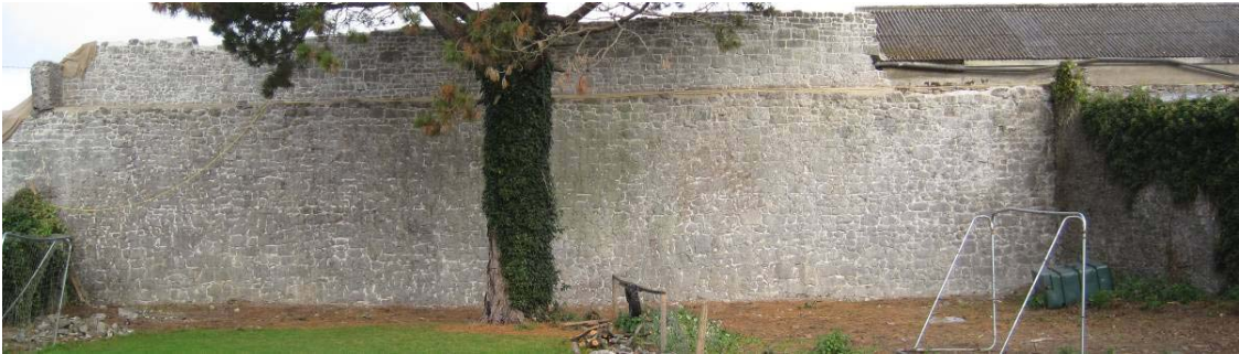
Fig 22 Section B-2010 (Gazetteer 2.36) South side (Gerald Manton's garden) After conservation. Note replacement of stones in parapet.
