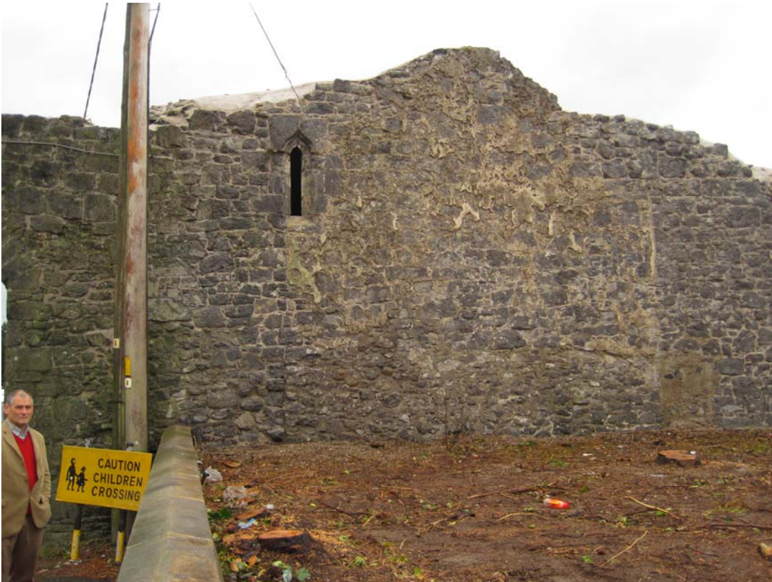
Fig. 13. Section A-2010 (Gazetteer 2.01) South side. View of newly discovered window in south wall of Currikeen Castle, after conservation.
